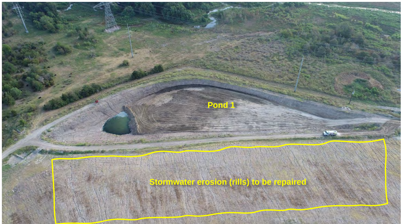
Photo 1 - Site A Landfill Pond 1 – Waste has been removed from pond; Evidence of stormwater erosion issues (8/10/2023)
