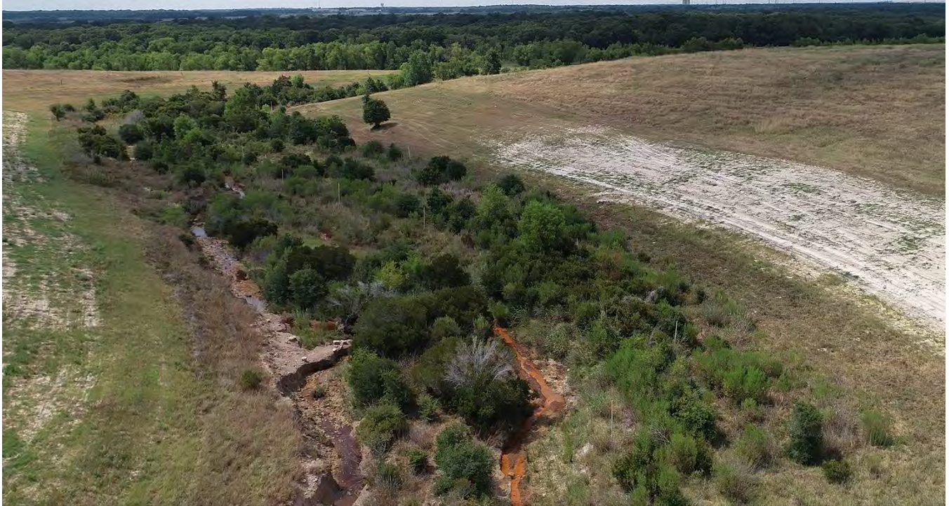
Figure 3 – Seep 9A area before mitigation
