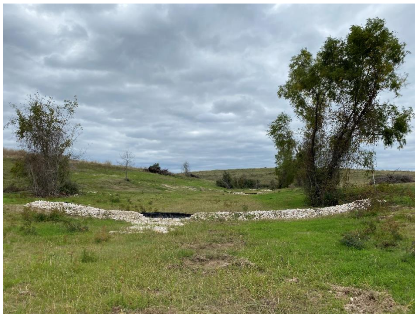
Figure 2 – Lower part of Seep 9A drainage, reclaimed in 2023 (view south, 11/21/23)
