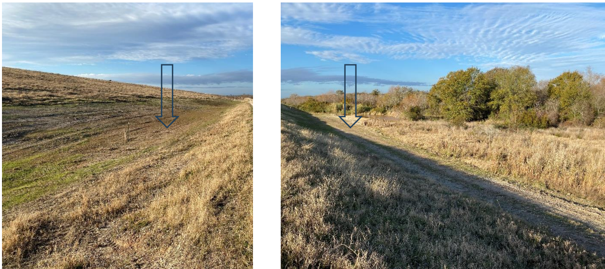
Figure 4 – Seep1A – buried French drain (left) and buried gravel bed (right) (view southwest, 12/20/23)
