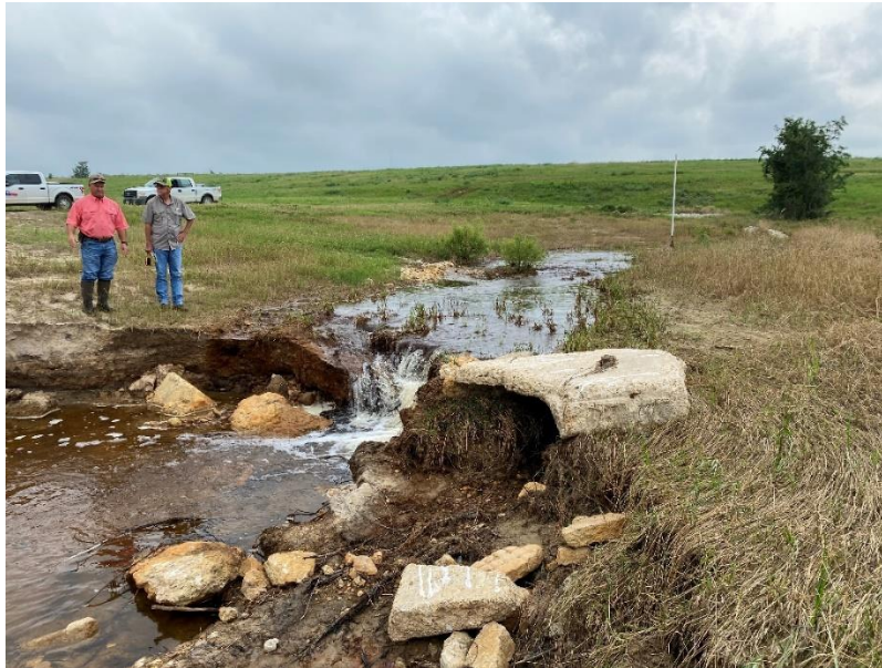
Figure 5 – Seep 9A – Erosion at lower end of drainage (view south, 05/28/24)
